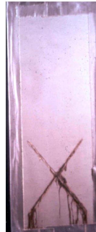
Three-Coats U-104 On Pre-Rusted Panel After 14,000 hrs in Salt Fog
